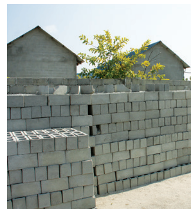
The waste management centre under construction on Vaikaradhoo Island, Maldives © Hanying Li
